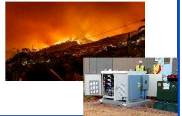
Utility Operated DERs during PSPS
